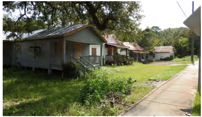
These boarded up and derelict houses are illustrative of many areas of Thomasville. More should be done to limit and stop the increase in these types of properties.
