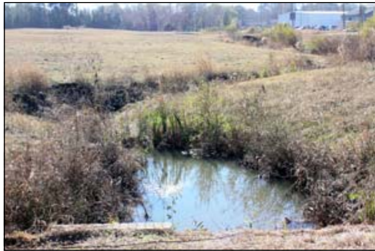
The trail will cross Oquina Creek on Wolf Street and will require either a timber bridge or an open bottom culvert adjacent to the street.
