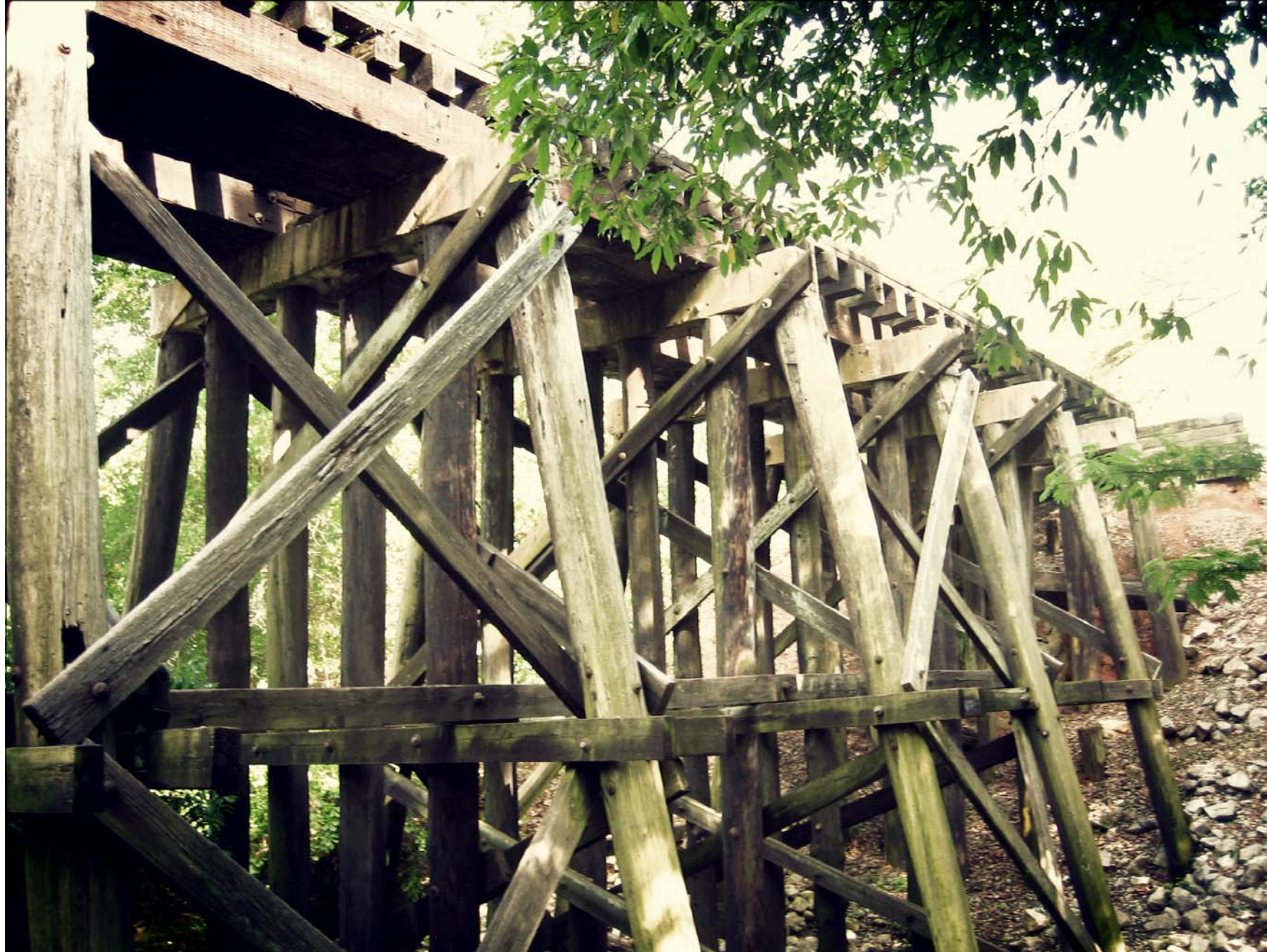
Railroad Trestle in Thomasville A railroad trestle crosses an Oquina Creek Tributary at a proposed trail alignment location.
